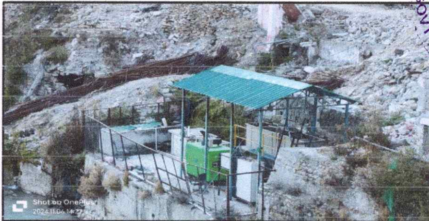
0.01 MLD STP near Badrinath Temple
